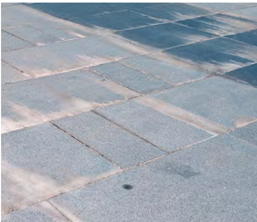
Efflorescence manifests as unsightly white patches on tile surfaces
