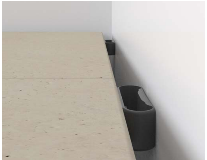
Gap between pavers and wall
